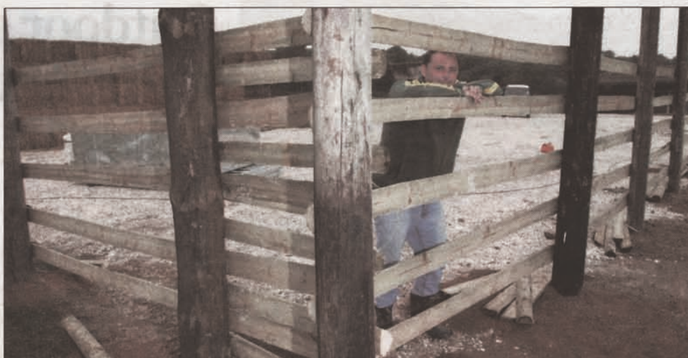
The corral is made of a crushed chalk base surrounded by posts and rails to a height of two metres.
